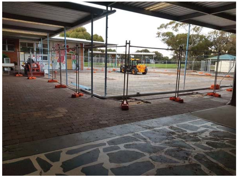
During the term 2 break we said good bye to the old library, making way for our new learning spaces expected to commence being built at the end of the
